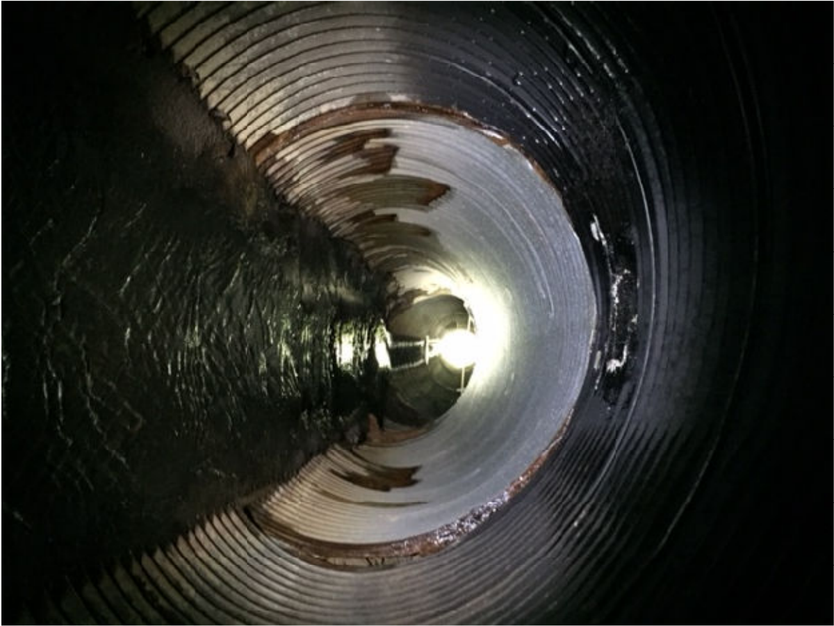
Failing bottom and joint
