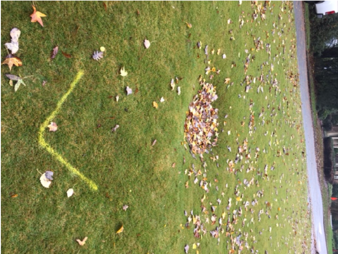
Sinkhole forming at 5113 Meadow Creek Drive
