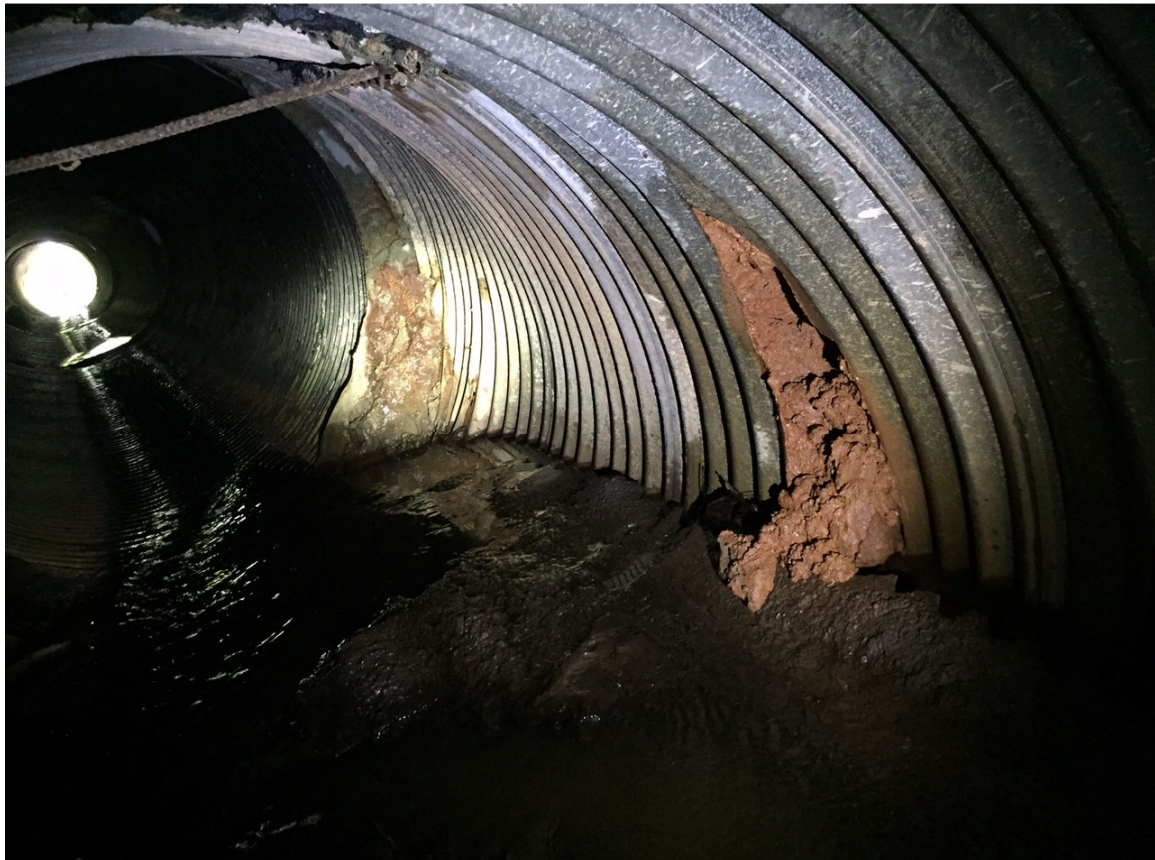
Pipe Failure under Sinkhole
