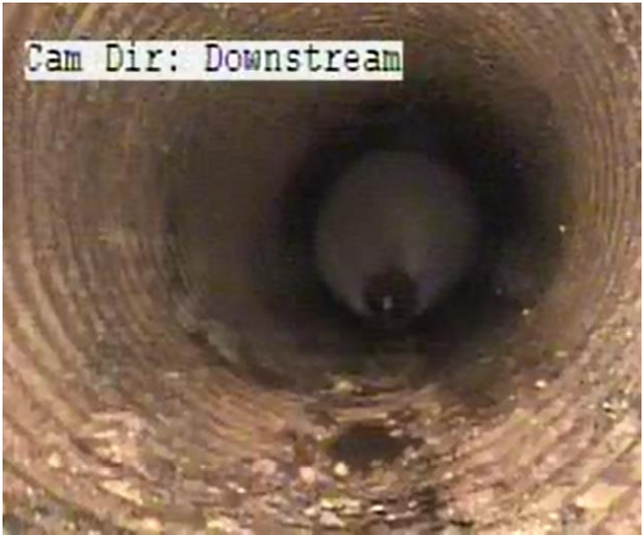
Missing invert in portions of 24" culvert
