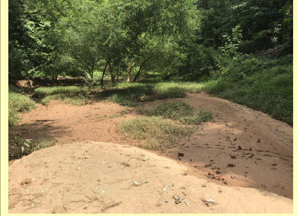
CITY - MAINTAINED PROPERTY SEDIMENT & GRAVEL DEPOSITED IN DETENTION POND
