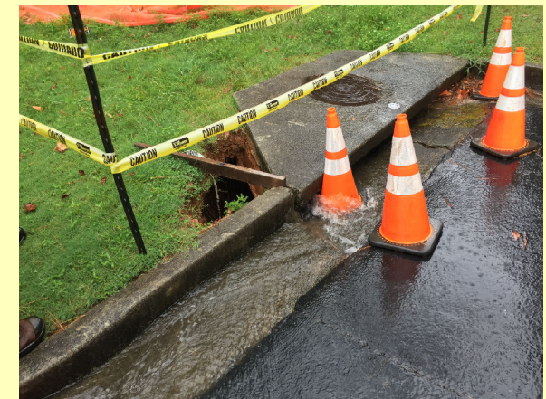
SINKHOLE EXTENDED TO CURB & GUTTER OF PARKING LOT
