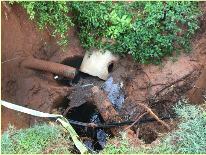
30 FOOT WIDE x 20 FOOT DEEP SINKHOLE COLLAPSED JUNCTION BOX
