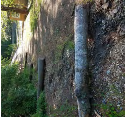
Evidence of erosion upstream of stormwater pond.
