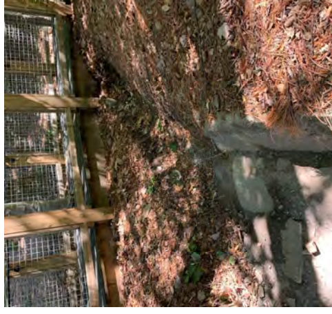
The culvert underneath the existing footbridge is full of debris, causing erosion issues.
