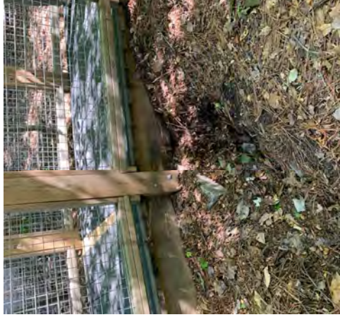
Because water cannot travel beneath the footbridge, moisture build-up is compromising the integrity of the wood.
