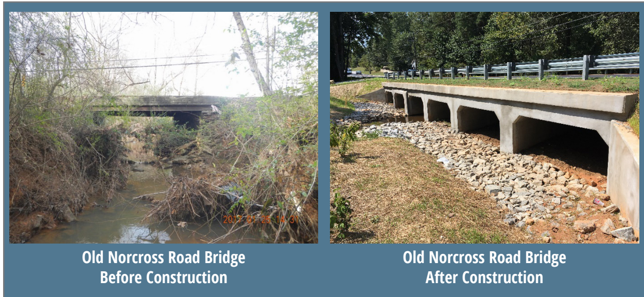
FIGURE 3: Dewberry developed the design, construction documents, and specifications, and provided permitting and bid assistance to replace the existing 19-foot span bridge on Old Norcross Road to address safety and hydraulic capacity deficiencies. Dewberry also provided construction management services, and construction was completed within budget.
