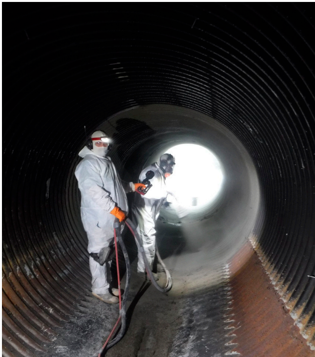
FIGURE 5: Application of CCCP for a design project completed by Dewberry for Gwinnett County. CCCP was selected to extend the useful lifespan of the existing CMP and increase the resilience of the stormwater system.
