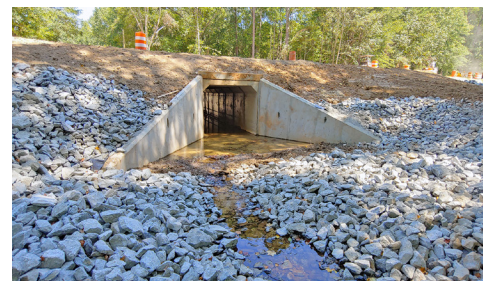
Fayette County, Stormwater Services
