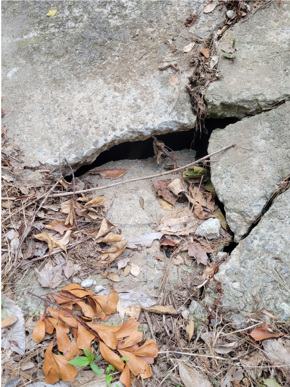
Sinkhole observed in driveway area Above 30" CMP
