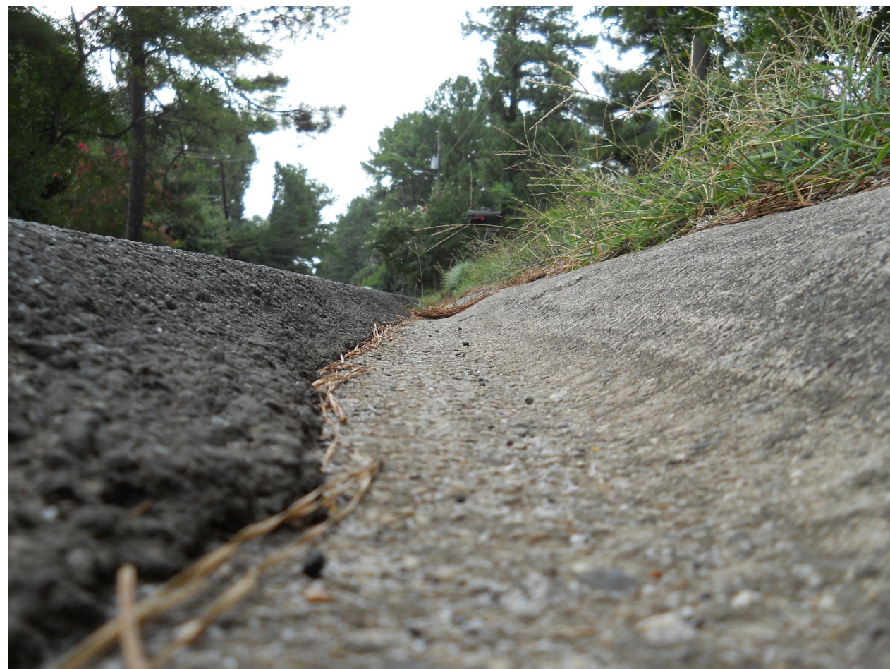
Pavement Buildup at Gutter on Happy Hollow Road
