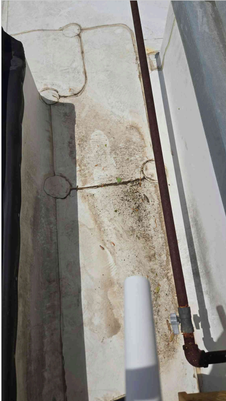
Condensate Pools on Roof.jpeg
